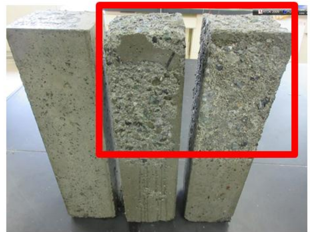
Figure 10 Promotion of the peeling damage of the coating area by surface impregnation materials
