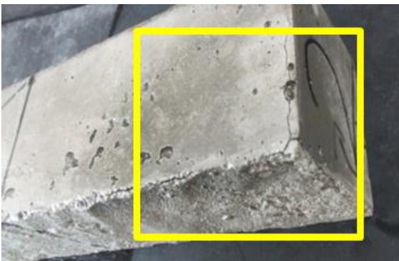
Figure 8 Initial cracking in the corners-cut square portion
